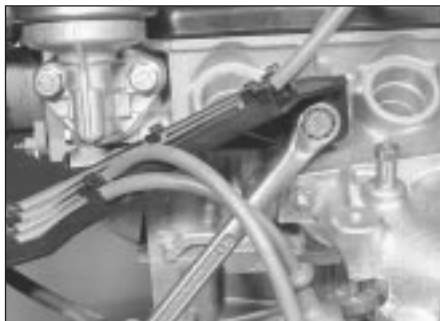
7.6 Unbolting HT lead support
